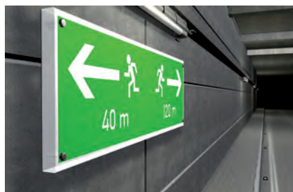
Emergency exit signs in tunnels
